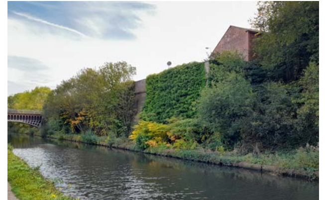
Plate 2.48 The retaining wall to the Corporation Yard along the New Main Line covered with vegetation
